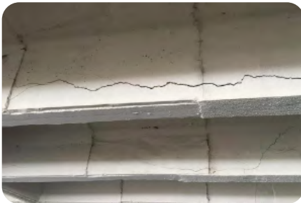
Beam with cracking
